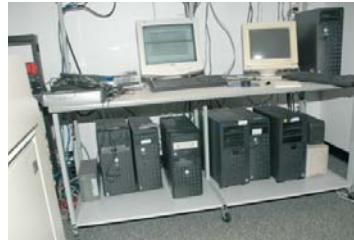
VIEW OF DELL SERVERS- MICHIGAN
