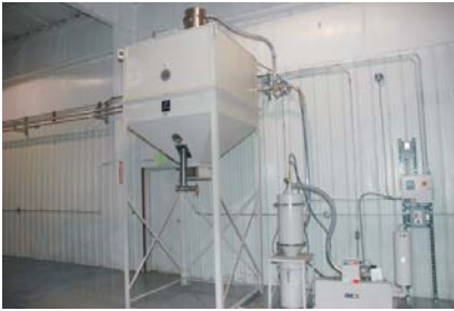
AEC SURGE BINS & RESIN PUMP
